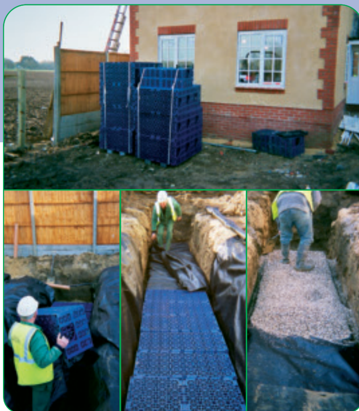
Domestic AquaCell soakaway
